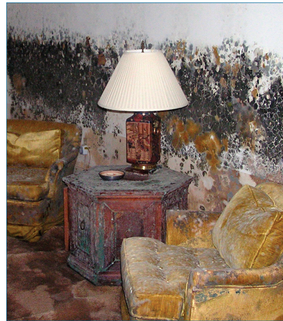
KEEP OUT Mold contamination in New Orleans has rendered thousands of homes unsalvageable.
